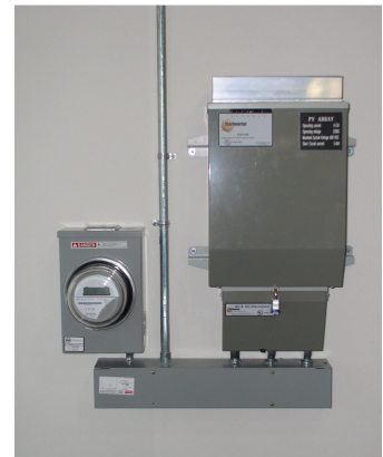
Fig. 3: PV Power inverter meter at the Oregon Office of Energy in Salem, Oregon.
